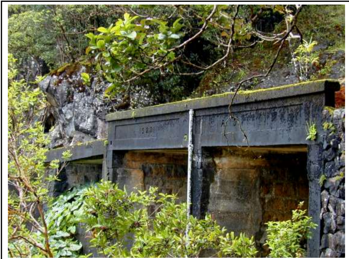
Kikokiko Bridge (1922), EMI mauka Route between Pāpaʻaʻea and Kopiliʻula i uka (Photo No. KPA-1397)
