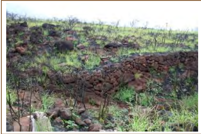
Figure 3. Stone-lined wall of Lahainaluna Ditch, Crossing Gully in Halaka'a, North of Kaua'ula Stream (Photo No. KPA-C5129).
