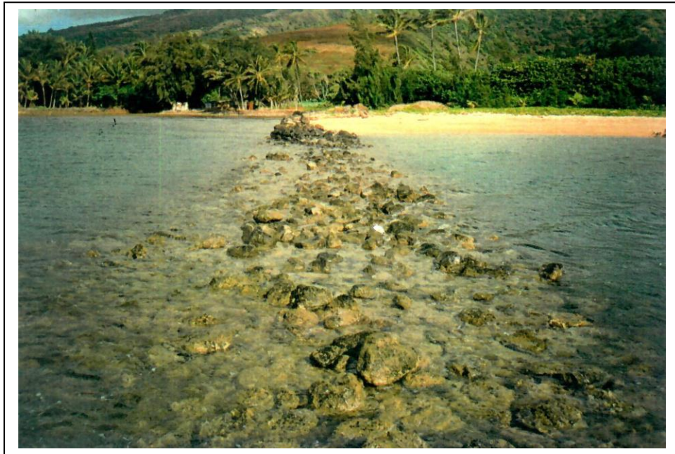
Figure 4a. Ipukaiole Fishpond Wall Prior to Undertaking Restoration Work in 1991 (standing on the western side of the wall, back to the ocean, looking towards the shore; Kainalu Stream on left)
