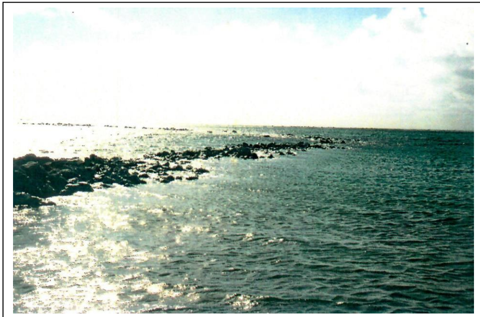
Figure 4b. Ipukaiole Fishpond Wall Prior to Undertaking Restoration Work in 1991 (back to the shore, facing out to the ocean; looking along the western section of the fishpond wall with outer wall continuing to the east)
