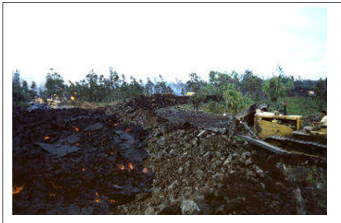
'A'ā flow has just reached the barrier built between Kuki'i and Kapoho. (Public domain.)
